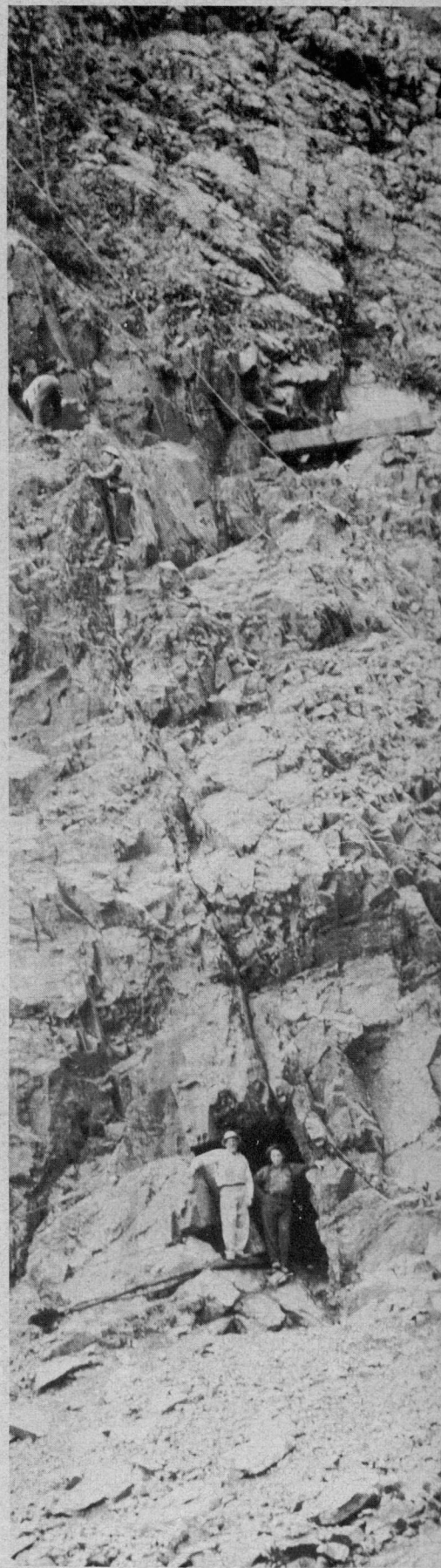
Jack Long and Earl Rider, a worker, stand in the tunnel mouth to show its size. Notice the ropes and men working higher up on the sheer cliff wall.
