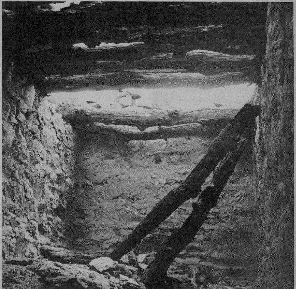
Tumbled roofs and well-preserved walls are all that remain of Fort Crittenden.
